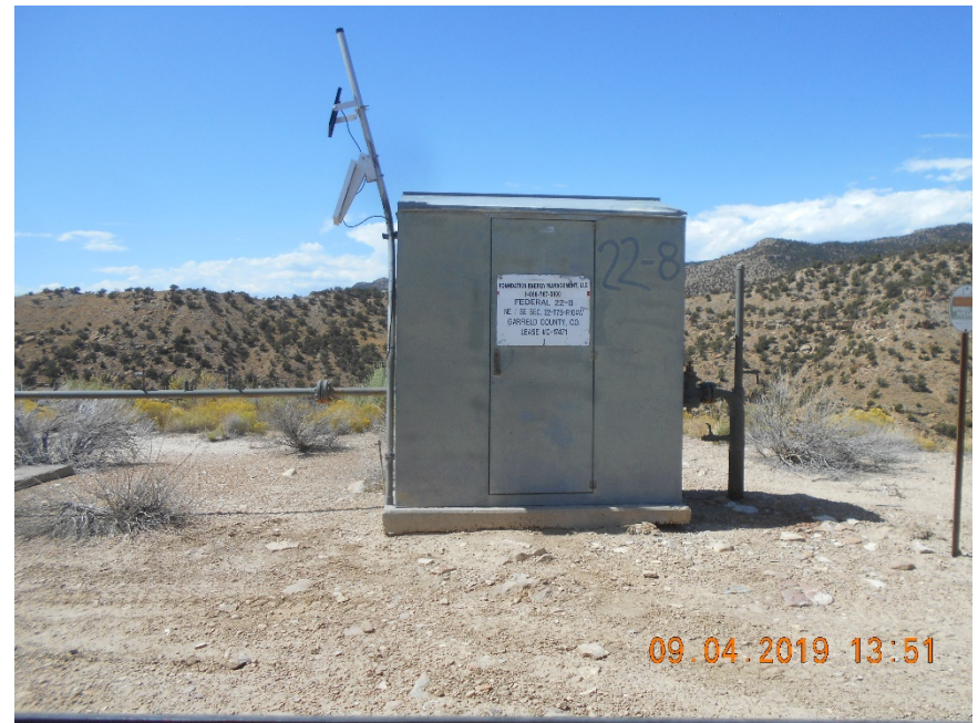
Meter housing with sign
