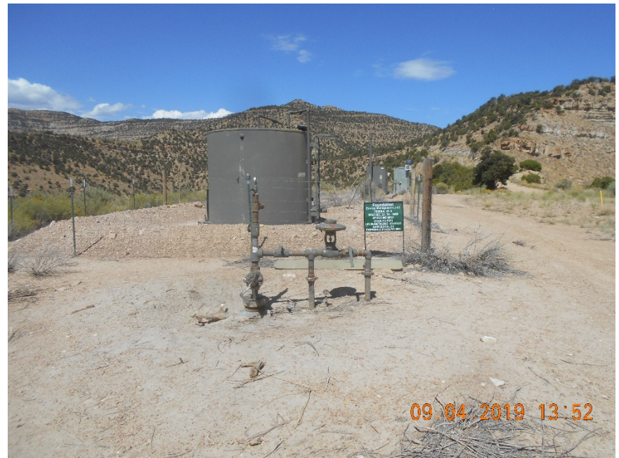
Wellhead with sign
