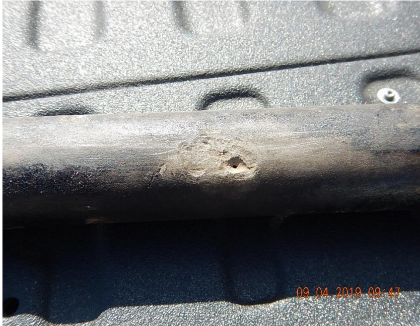
Failure point identified; External corrosion hole found. Coating has been removed.
