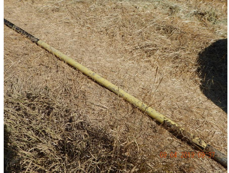
Section of flowline removed (Yellow Jacket); Coating has been stripped back to expose corrosion hole.
