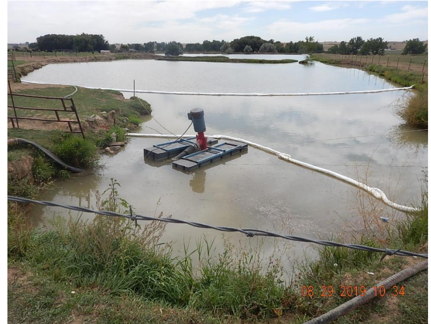
Spill response in progress; Impacted stock pond; booms deployed. View South toward Hillsboro Ditch.
