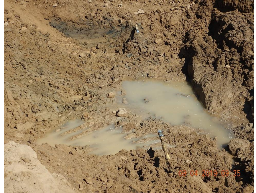
Cut ends of flowline in excavation threaded and bull plugged. Flowline is scheduled to be removed/ replaced.
