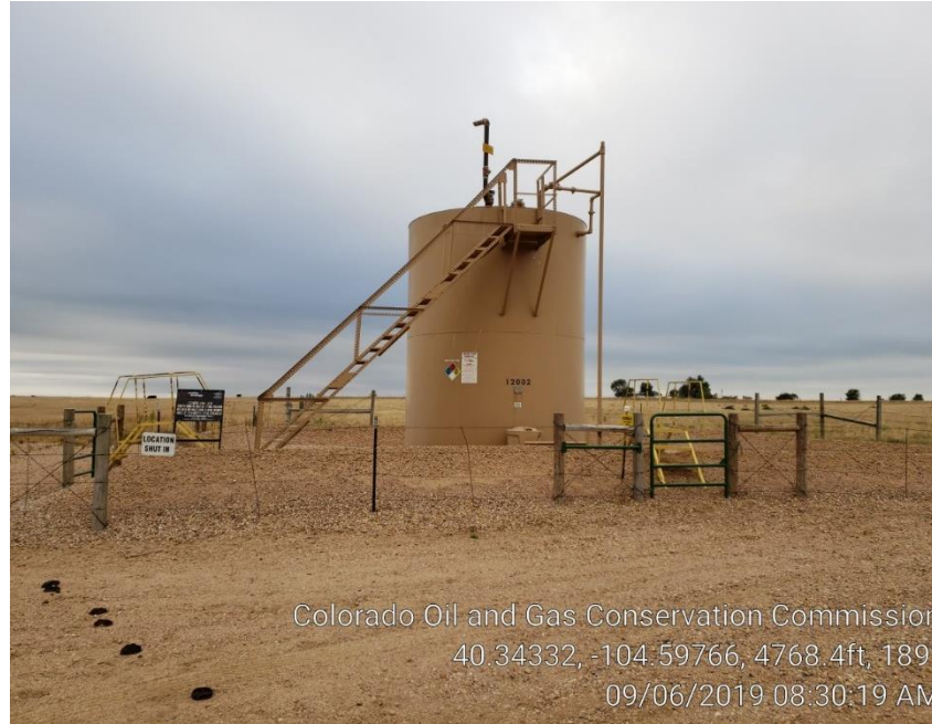
Photo #5 Tank Battery
