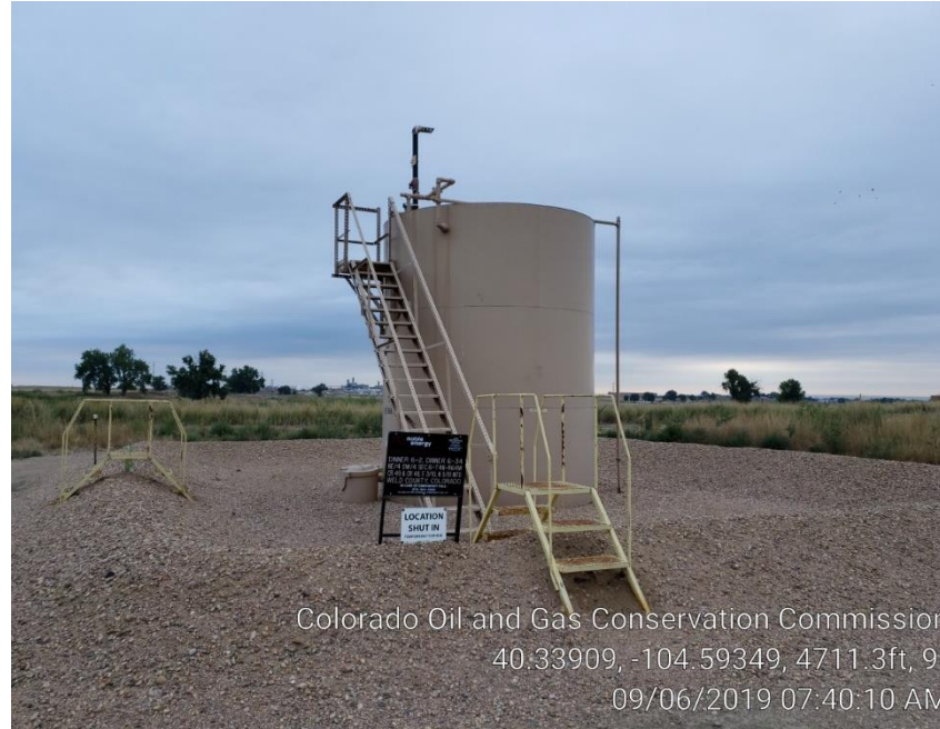
Photo #5 Tank Battery
