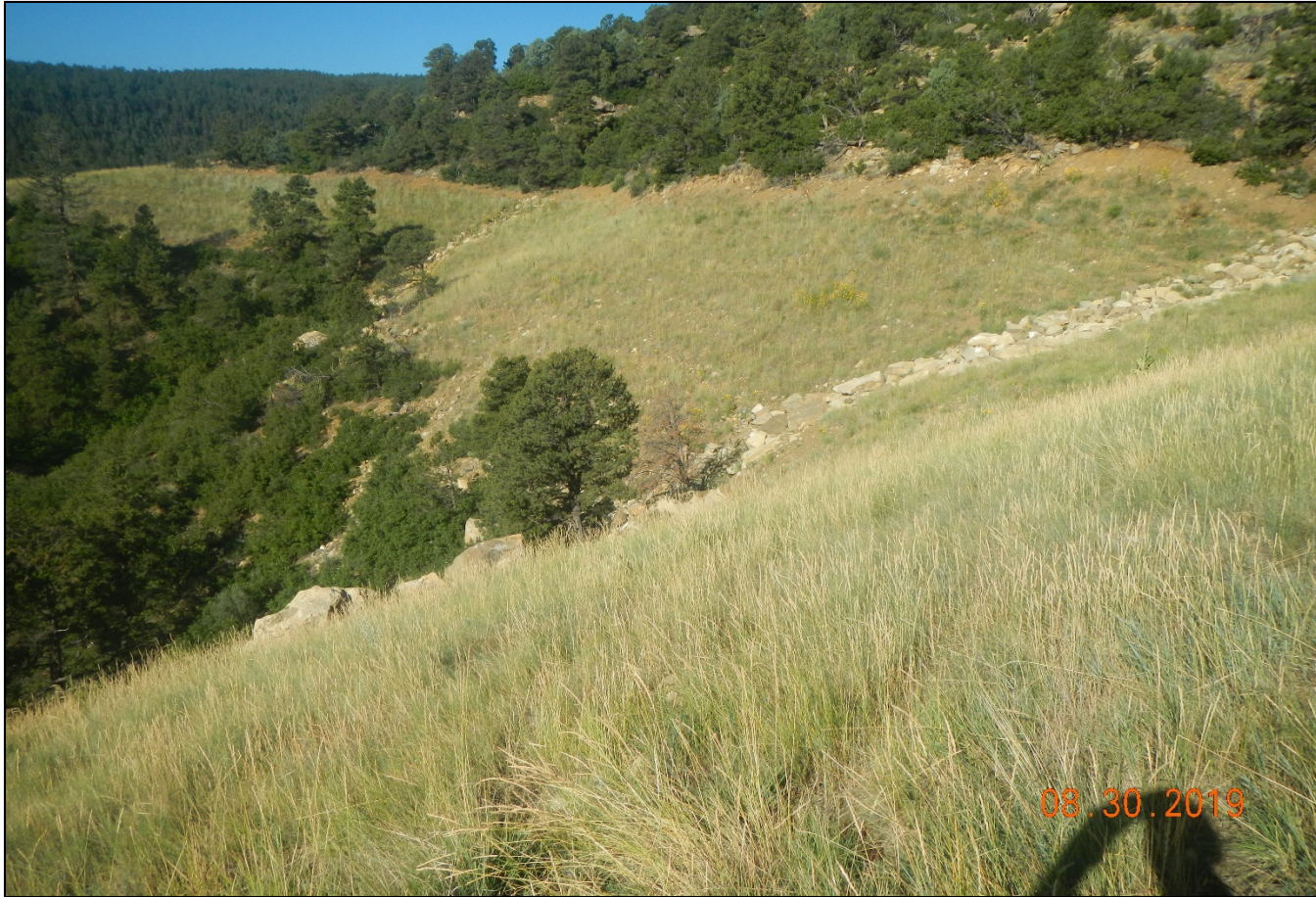
Photo 8. Facing northwest along the reclaimed access road. Rock rip rap was installed in the two drainages.
