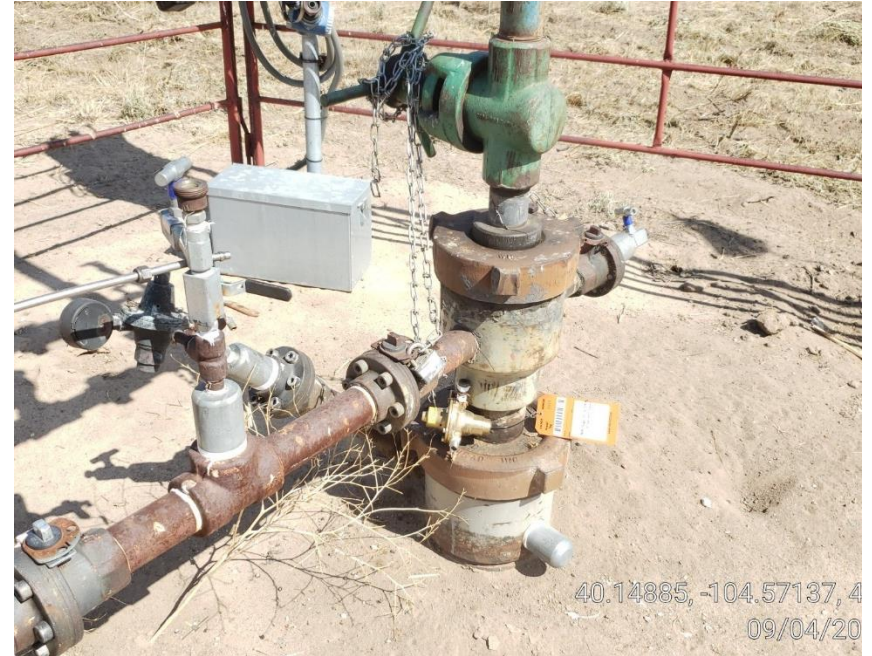
Photo #2 WH appears to be SI and LOTO for repairs
