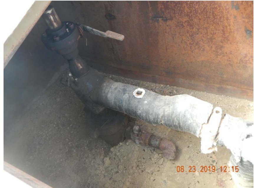
Photo 2. Photo of wellhead inside housing.
