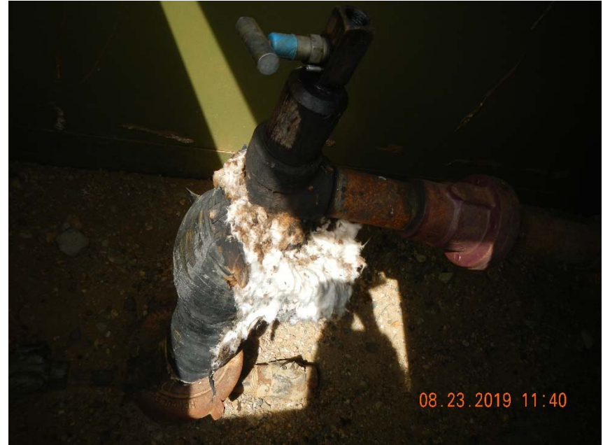
Photo 2. Photo of wellhead inside housing.
