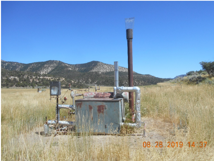
Separator and meter
