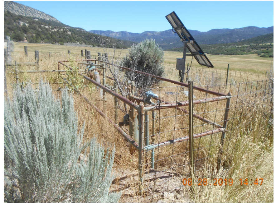
Flowline riser with fence at location entrance.
