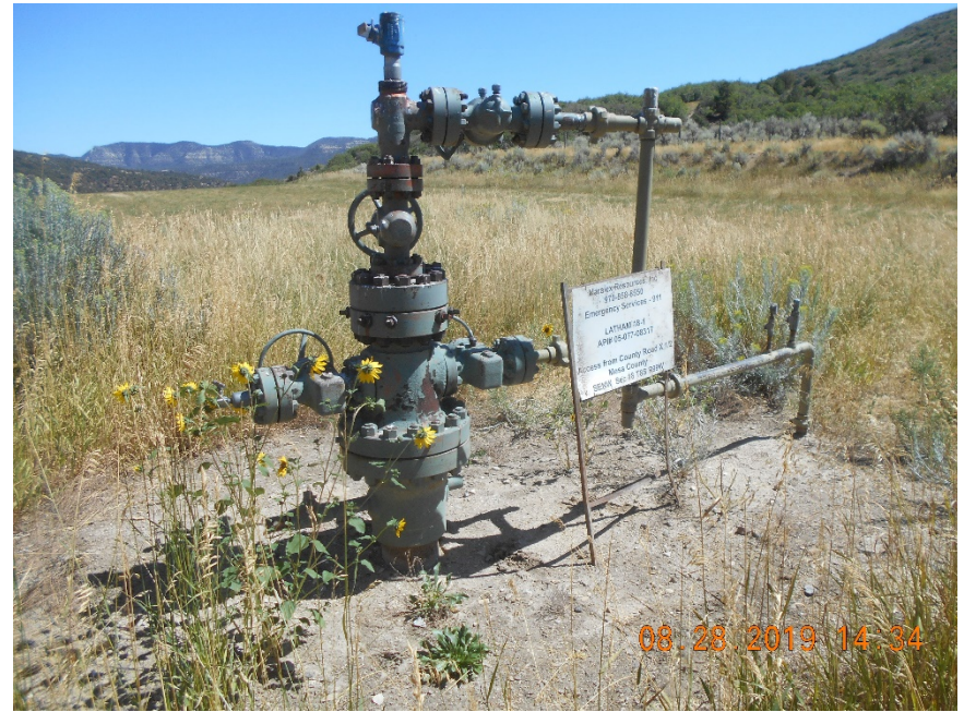
Wellhead with sign
