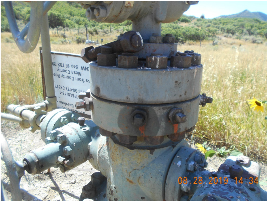
Audible gas leak at tubing hanger dog.
