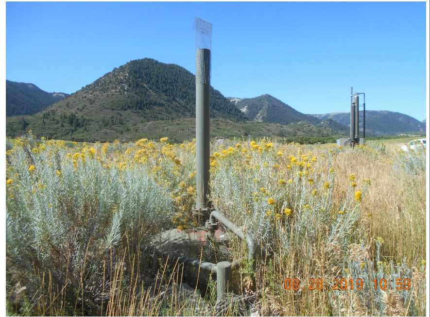
Partially buried tank with no berms or labels. Overgrown with vegetation
