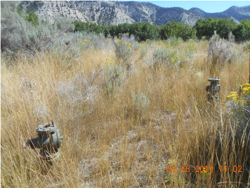
Multiple unused risers. Not locked out/tagged out. No blind flange on open end
