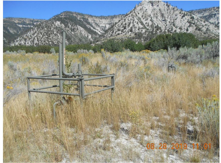
Unused riser in fenced area.
