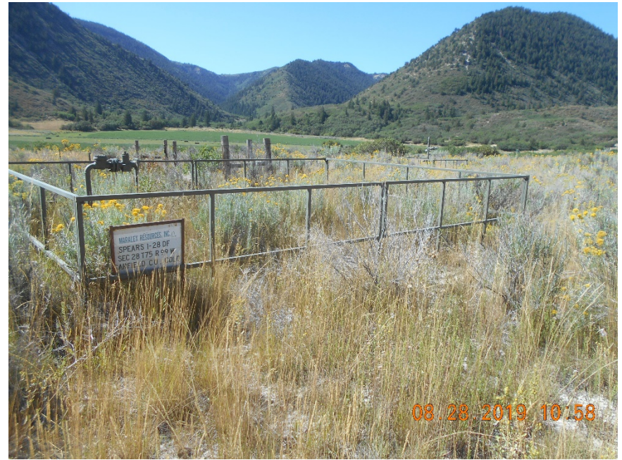
Unused riser in fenced area. Not locked out/tagged out. No blind flange on open end.
