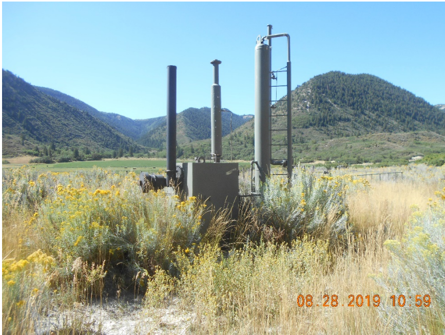
Separator overgrown with vegetation.
