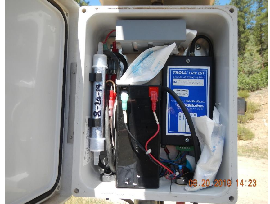
Troll Link 201 equipment enclosure with fresh desiccants.
