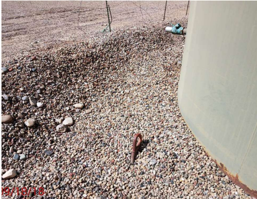
Previous inspection photo of dead man unmarked
