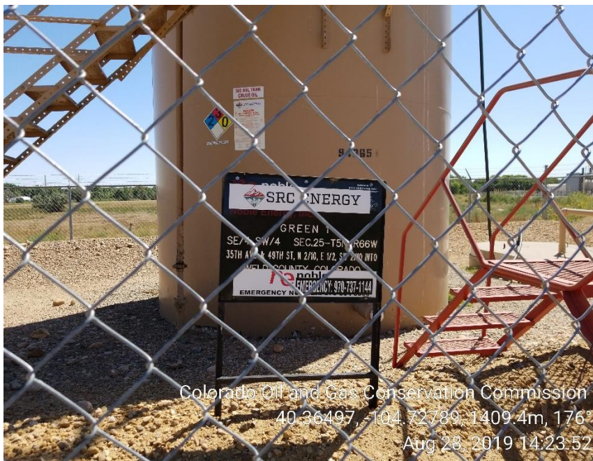
Photo 3: Tank Battery Sign
