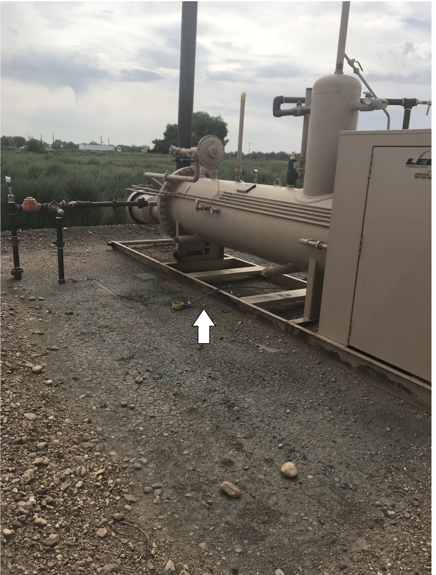
Counter 1AD & Dita 1A production facilities
