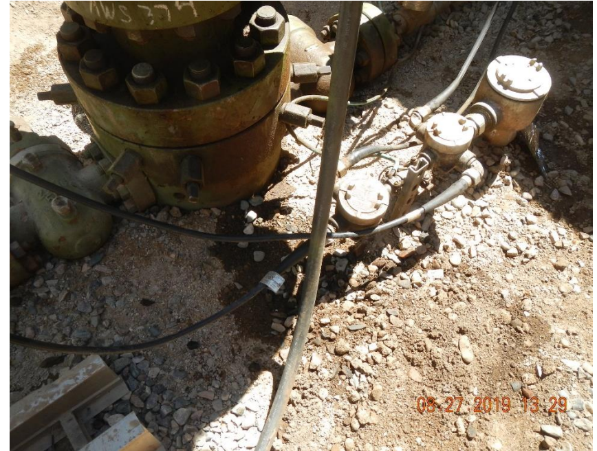
Stained/damp soil adjacent to well head.
