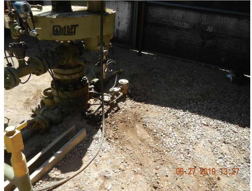
Disturbed area of soil and gravel adjacent to stained/damp area.
