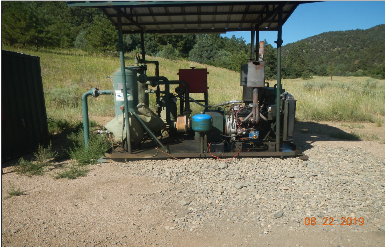
Photo 2. There is oil in the engine skid and staining on the surface.
