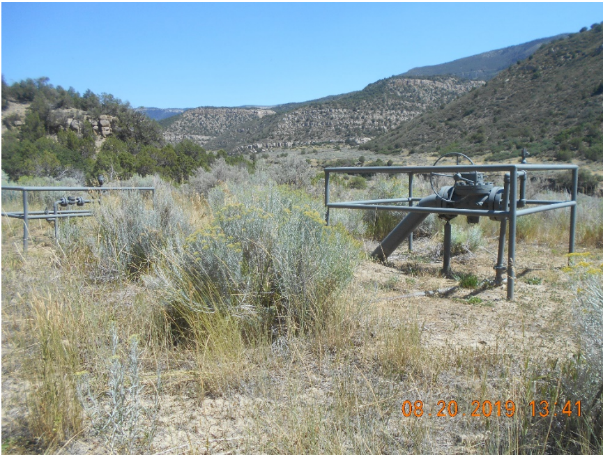
Flowline riser with fence
