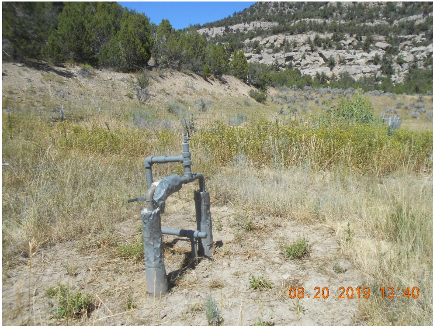
Pit with fence and netting. Flowline riser in foreground
