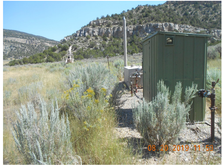
Separator and meter housing
