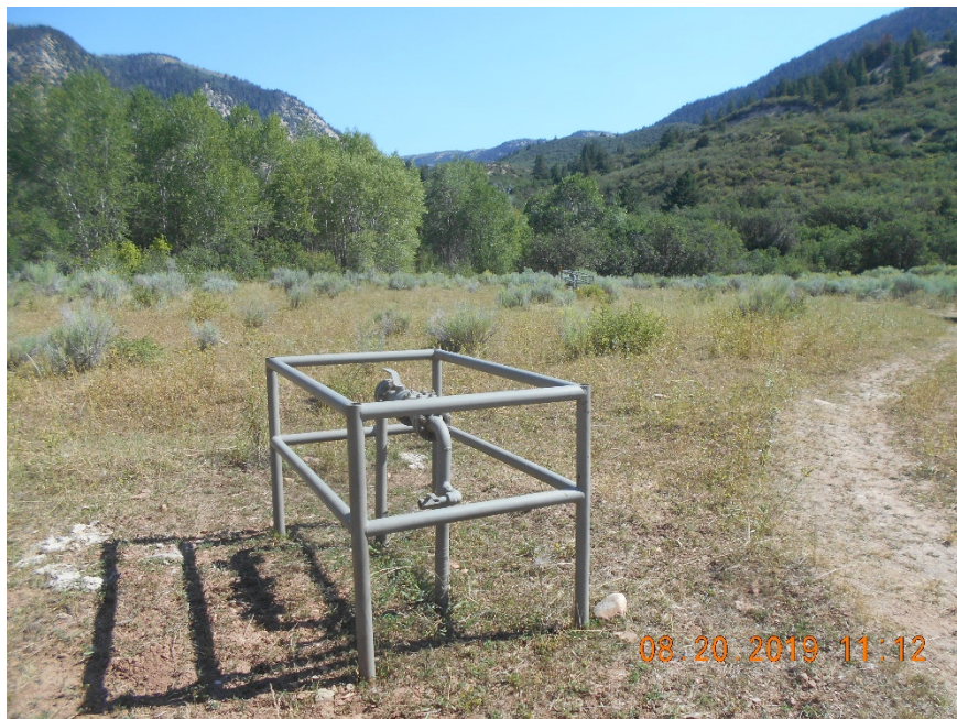
Flowline riser with pipe fence
