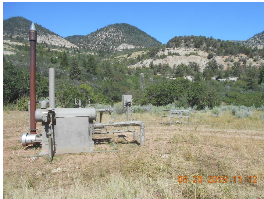
Separator and meter. Flowline riser in background.
