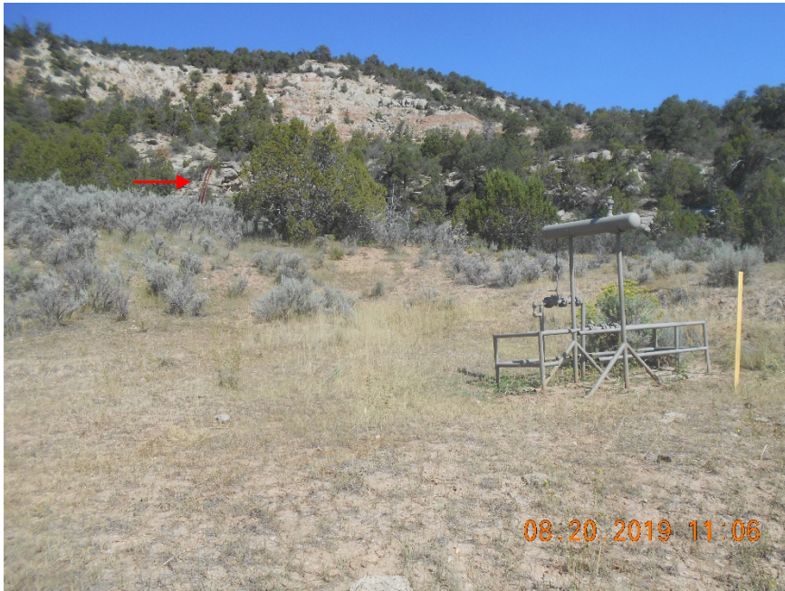
Flowline riser with fencing. Off location flowlines in background marked by arrow.
