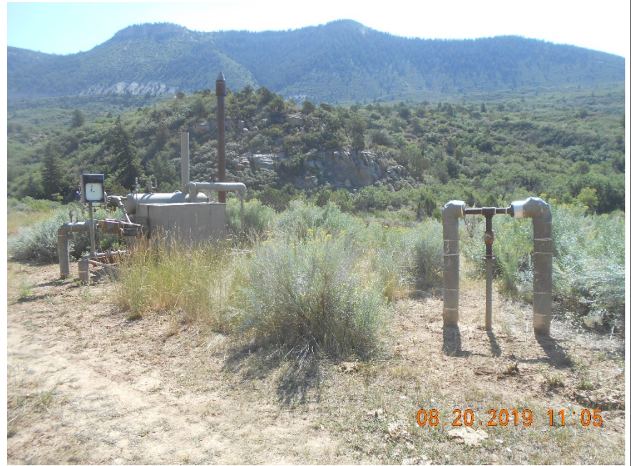
Separator and meter. Flowline riser.
