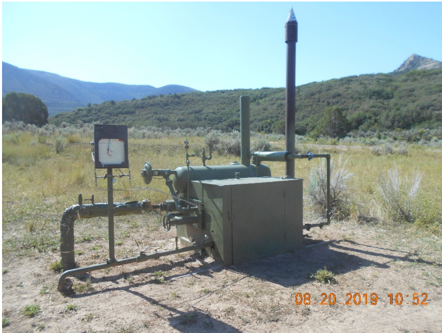
Separator and meter
