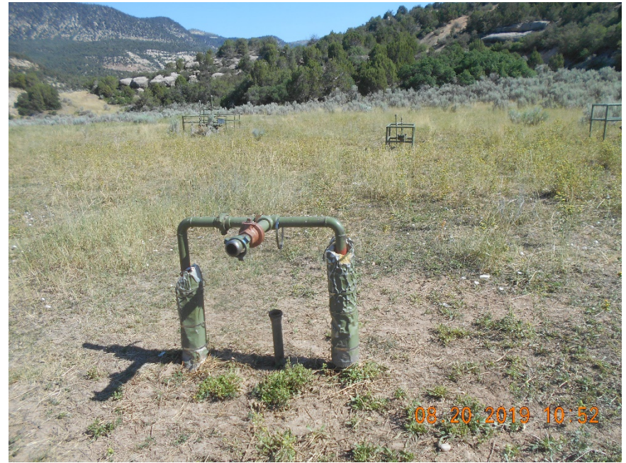
Flowline riser disconnected. Disconnected flowline risers not LOTO.
