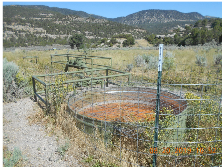
Blowdown tank with fence and netting. Flowline risers with pipe fencing in background.
