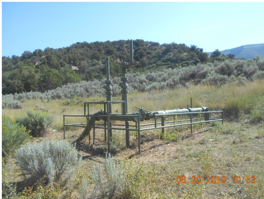
Flowline riser with fence
