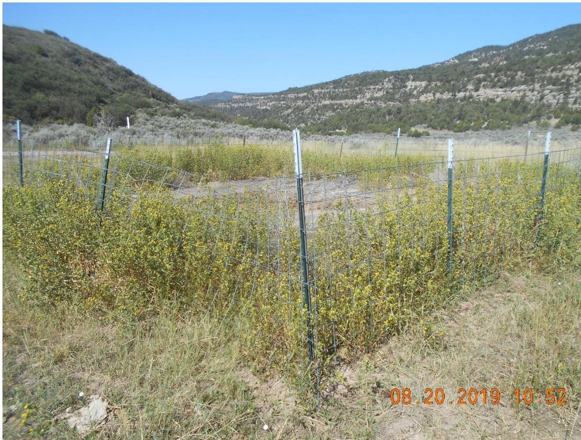
Blowdown pit with fence and netting. No weed control inside fence. Holes in netting.
