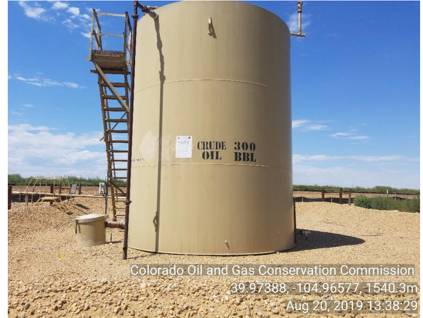
Photo 2 TNK BTRY placards have been installed.
