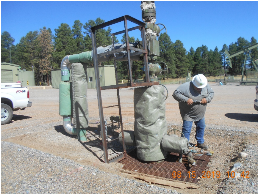
Injection wellhead with housing removed
