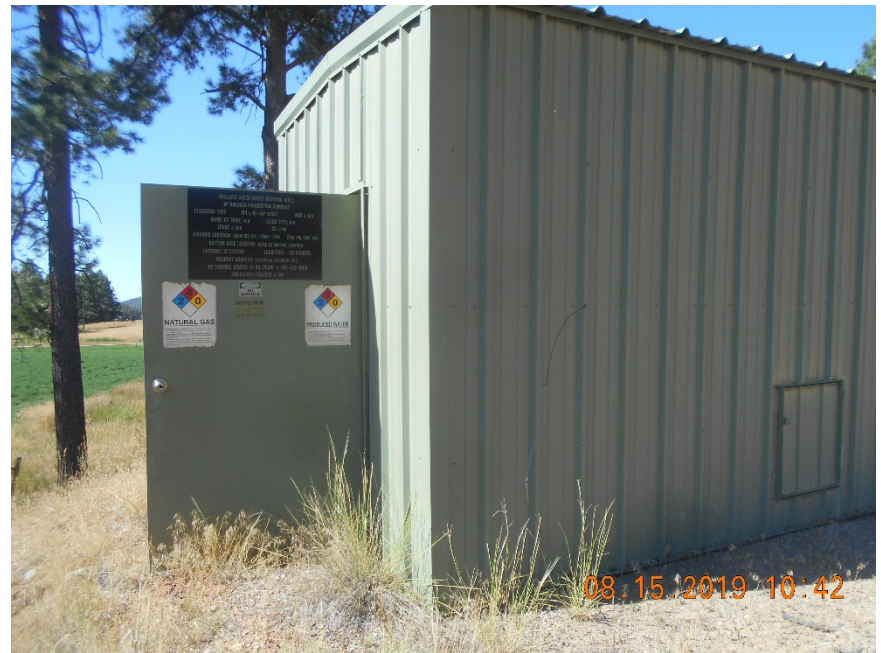
Injection well housing (removed) with sign
