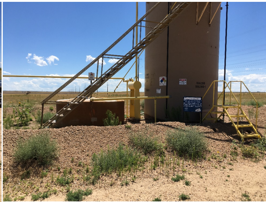
Tank battery looking south. 1 – 400 BBL crude tank and FG partially buried produced water tank. Note weeds.
