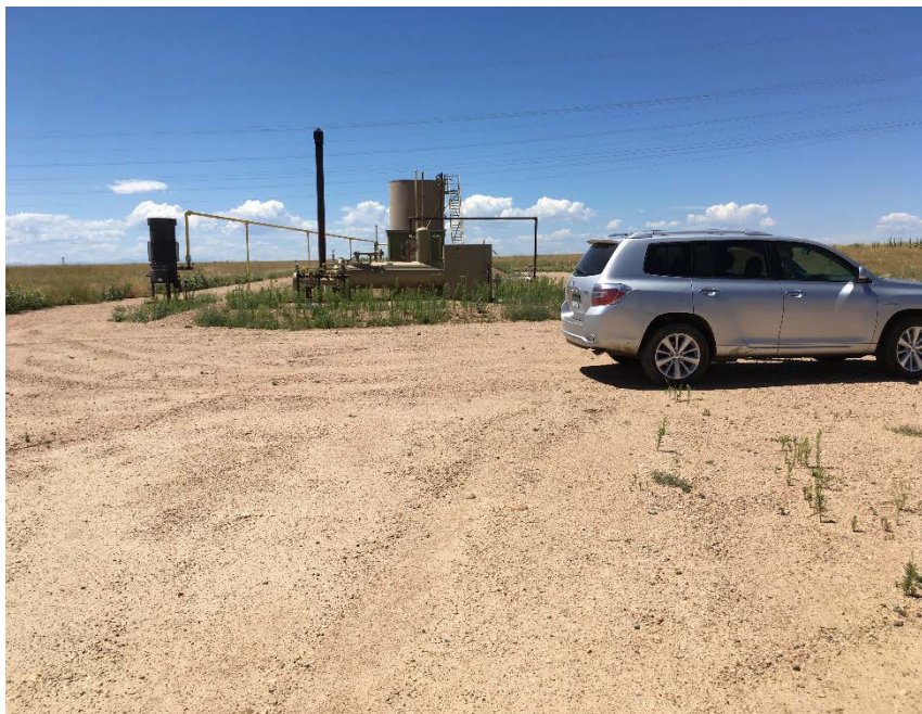
Tank Battery from wellhead. Photo looking west. Note weeds.
