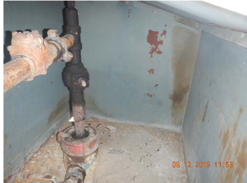
Photo 2. 0 psi on tubing, well shut in at time of inspection.
