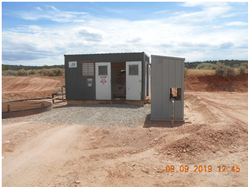
Pump housing. Meter shed.
