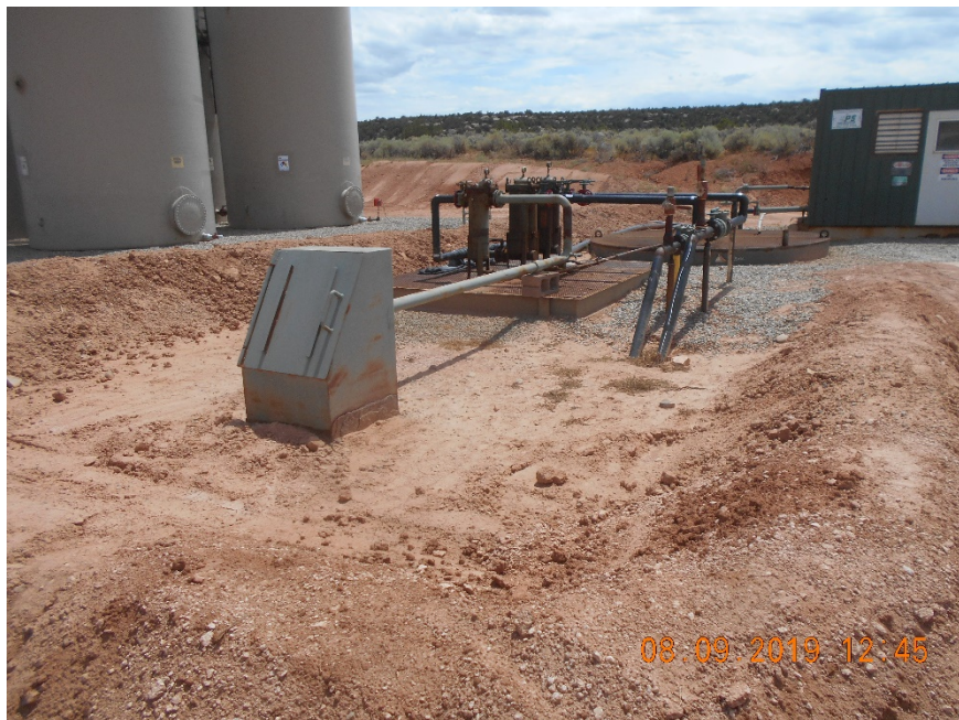
Loading station and Filter pod
