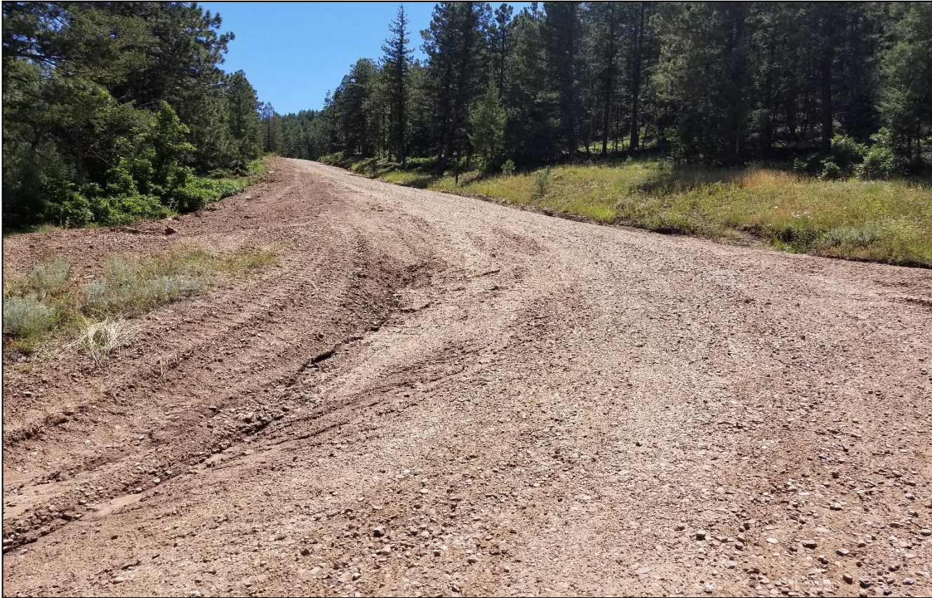
Photo 2. Vehicle ruts remain along the road which is a conveyance for stormwater erosion.
