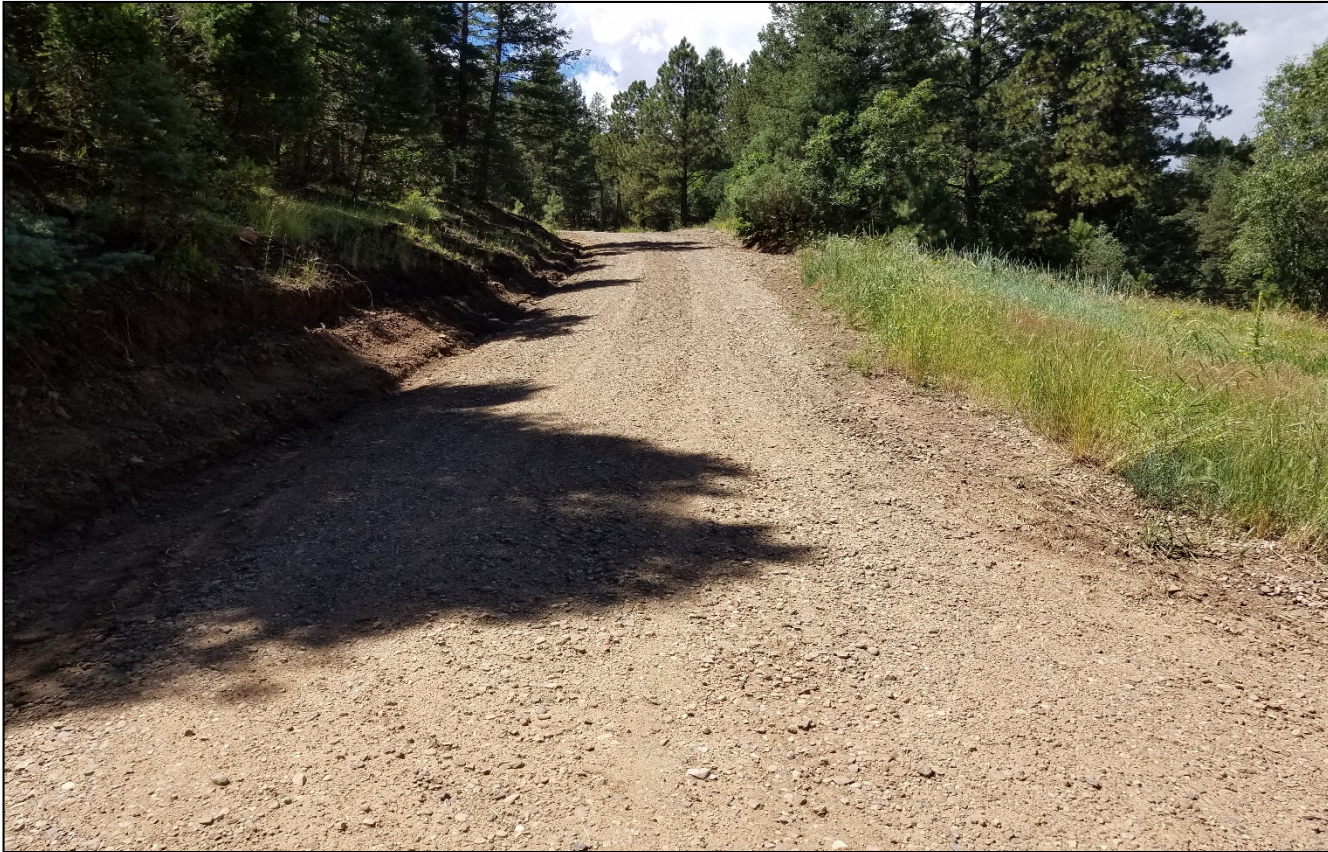
Photo 1. Vehicle ruts remain along the road which is a conveyance for stormwater erosion.
