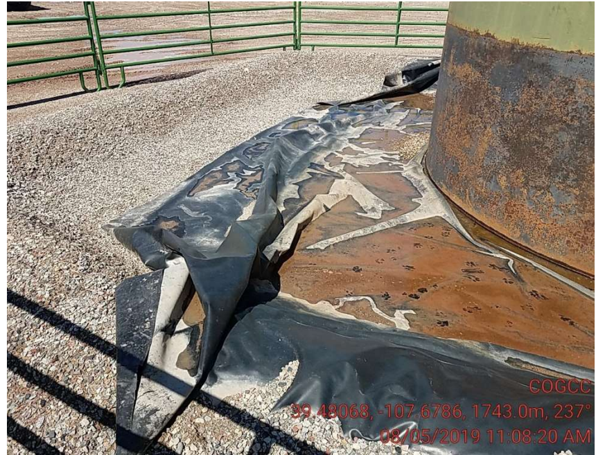
6 Braden head tank containment
