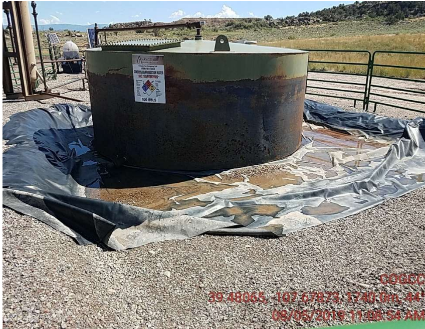
5 Braden head tank containment
