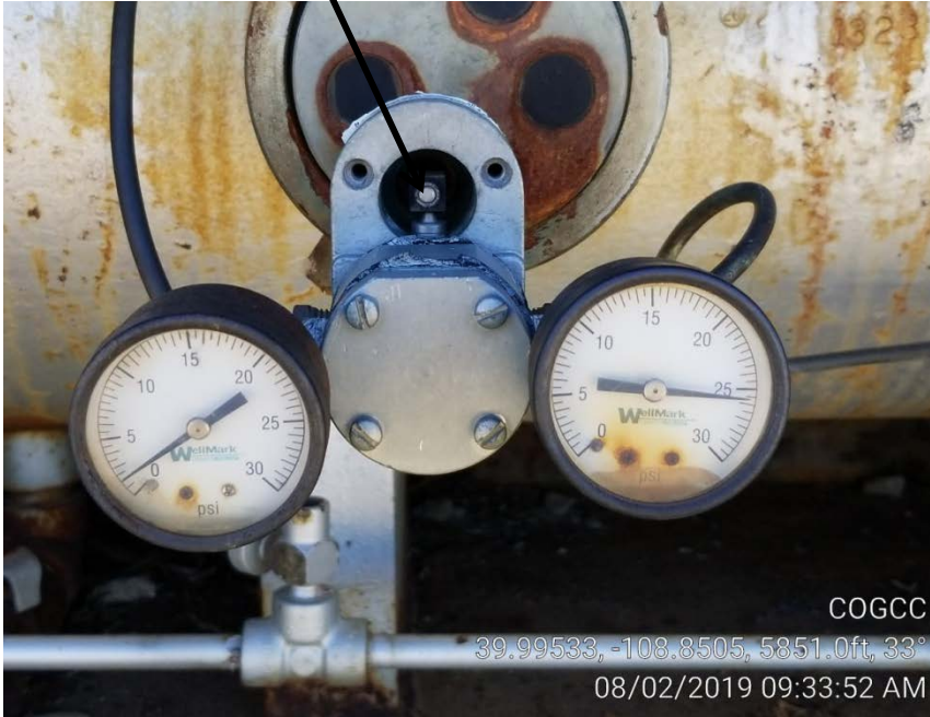
Photo 4. Separator gas leak.
