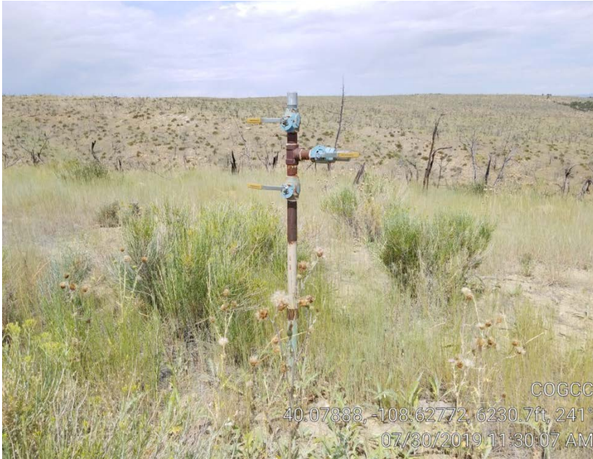
Photo 3. Gas liner riser.
