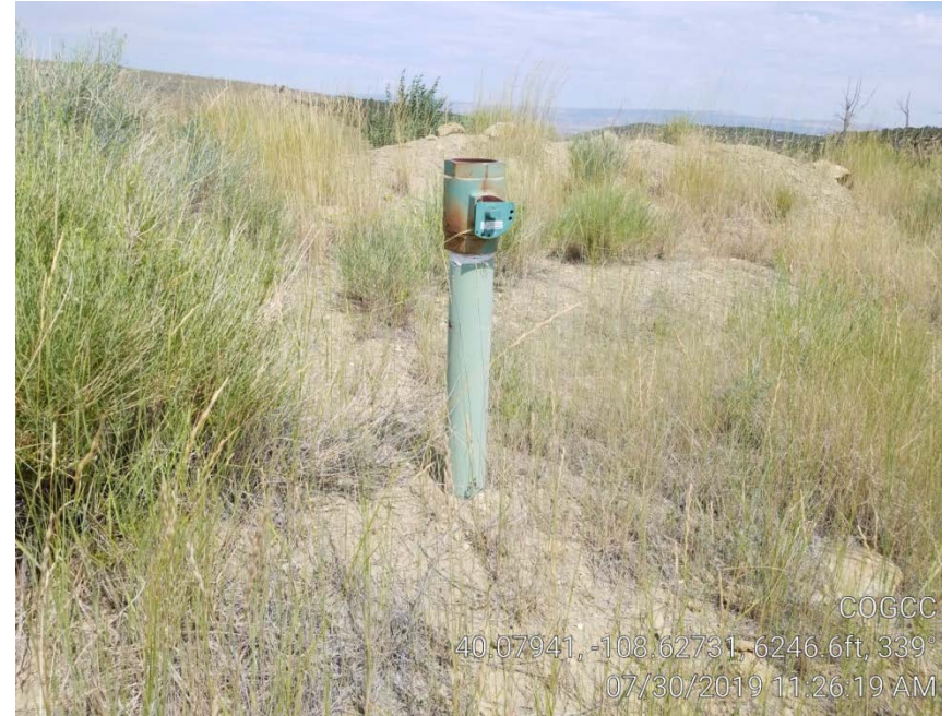
Photo 4. Gas liner riser.
