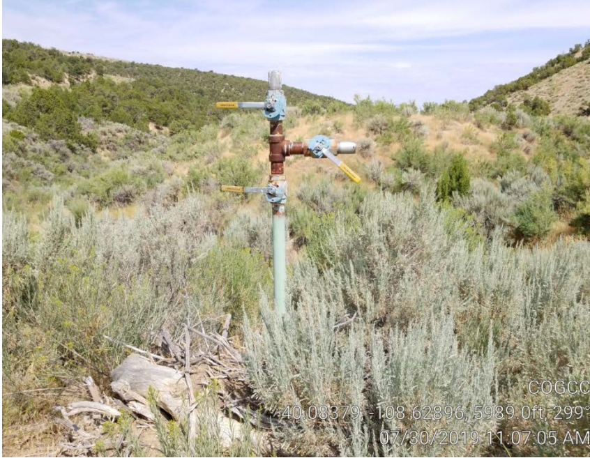
Photo 3. Gas line riser.
