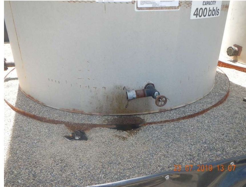
Photo #6 – View of the load out valve with stained gravel.
