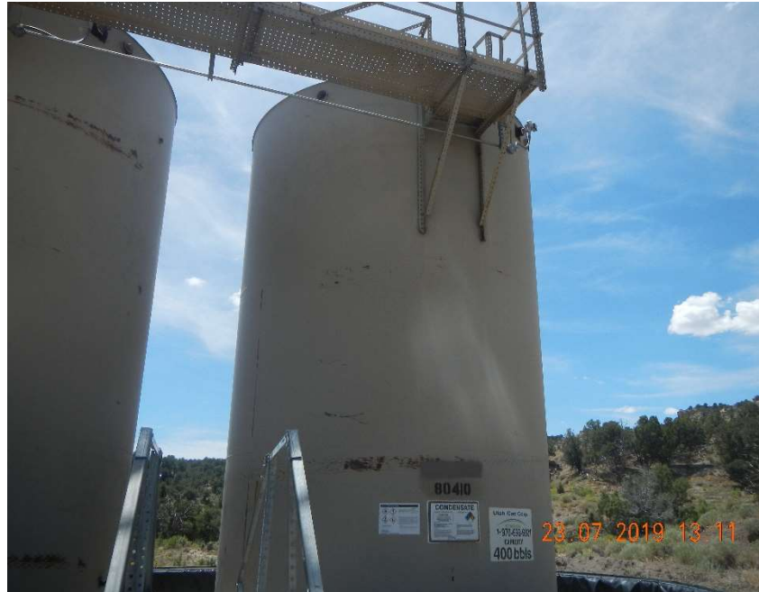
Photo #7 – View of open port on upper section of 400 BBL condensate tank #80410.
