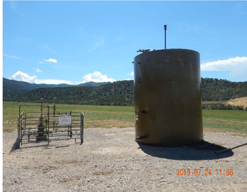
Photo #3 – Wellhead and condensate AST.
