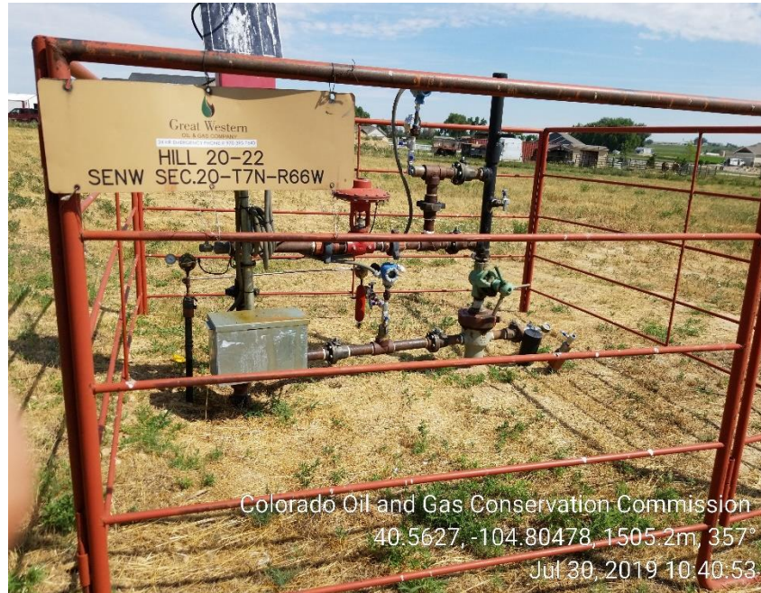
Photo 1: Wellhead; Sign contains emergency contact number
