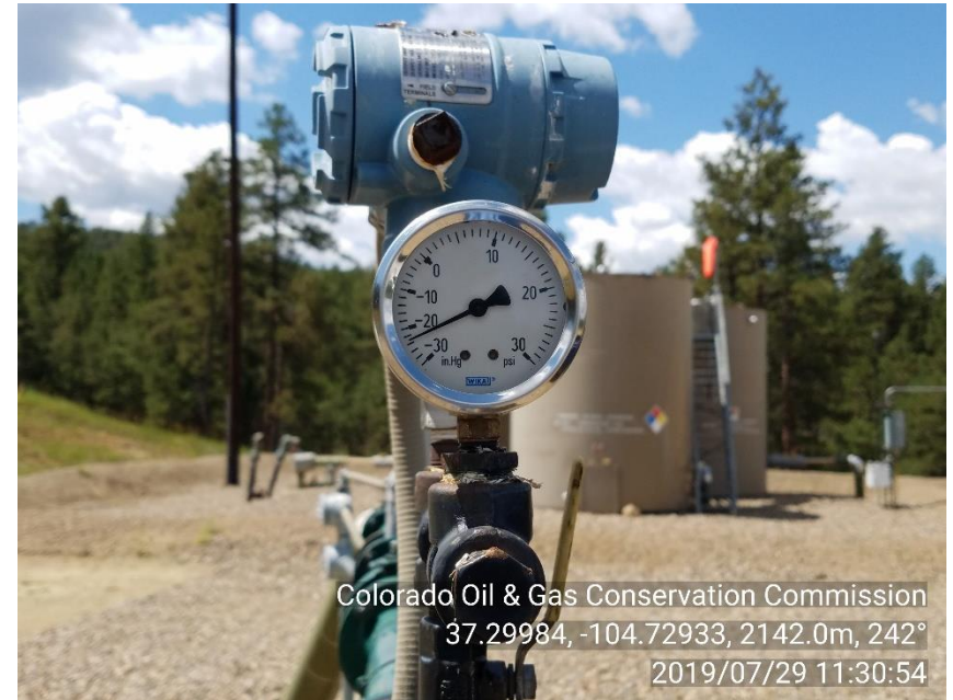
PHOTO 6: 0 PSI ON BACKSIDE BETWEEN TBG & CSG. MONITORED FOR 15 MIN. NO CHANGE
