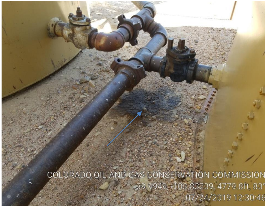
Pic 11 stained soil below valve
