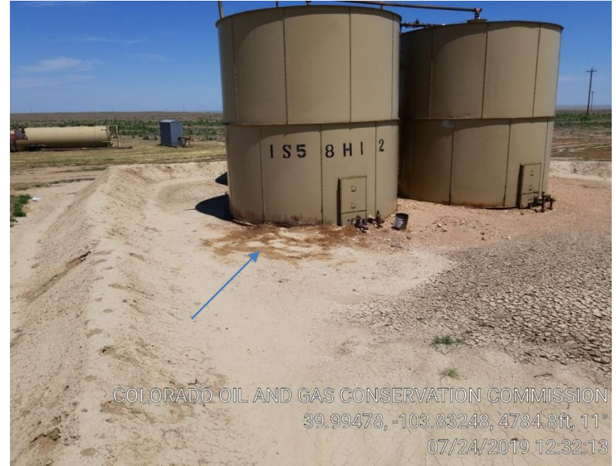
Pic 14 possible spill from tank
