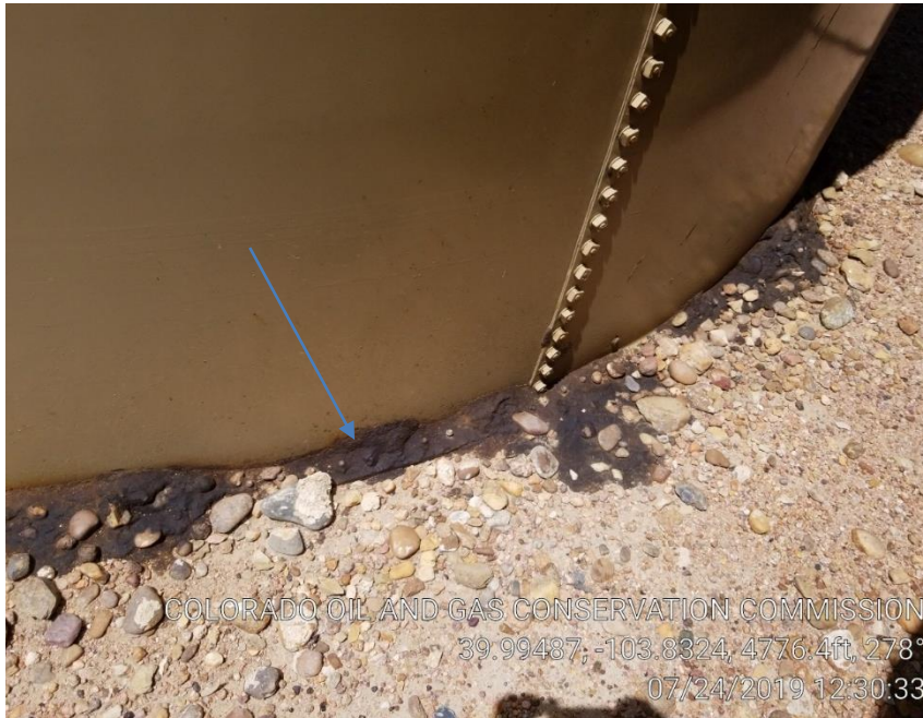
Pic 9 possible leak
