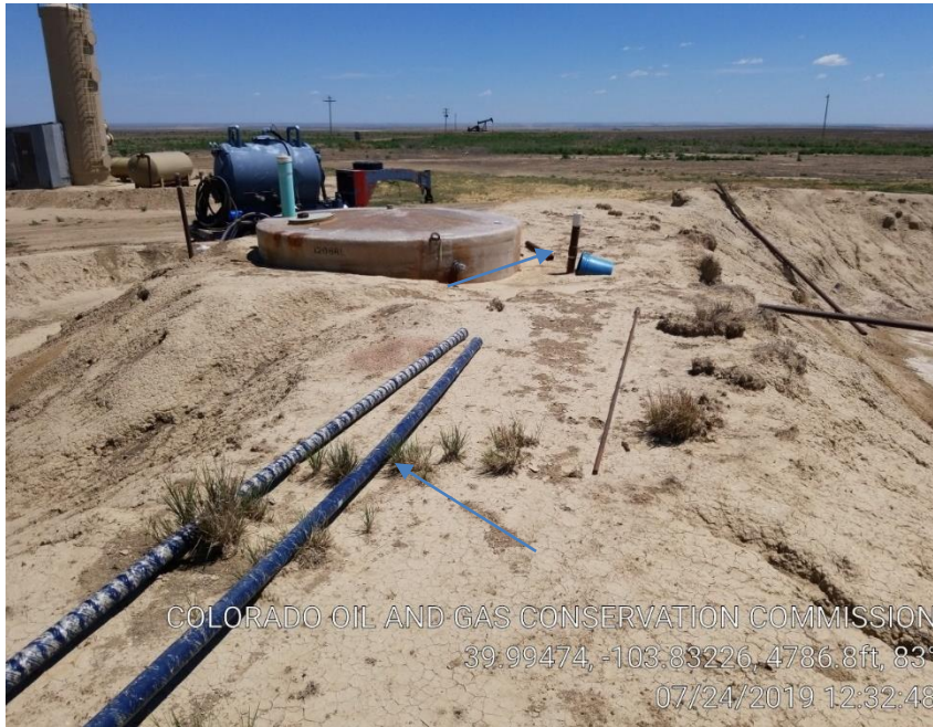
Pic 15 fiberglass tubing/trash around water tank
