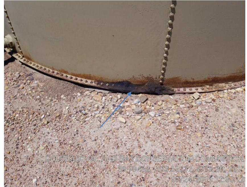
Pic 6 possible leak
