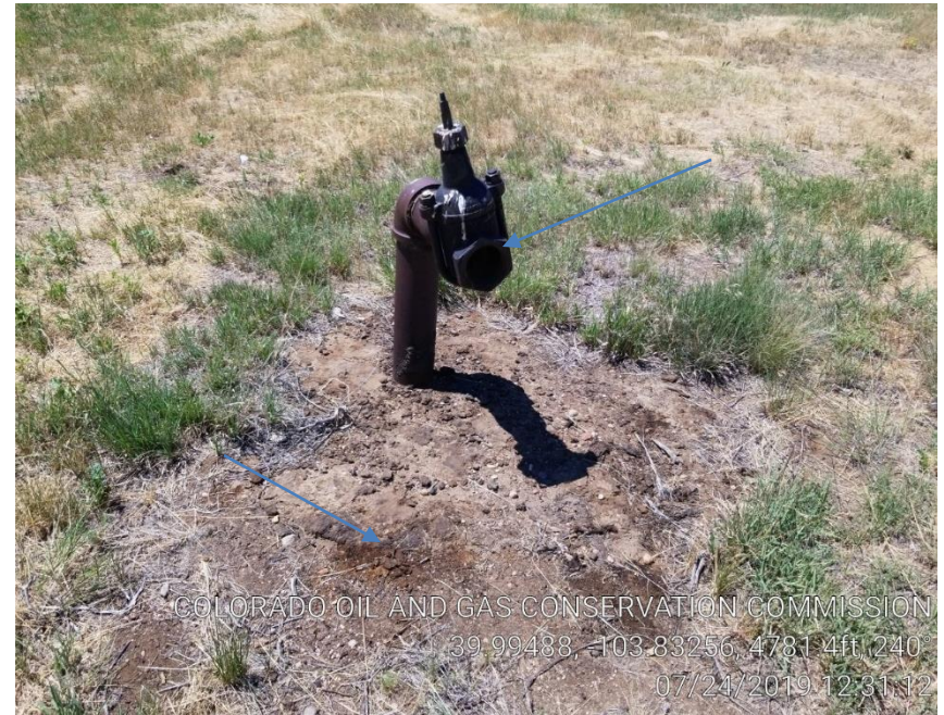
Pic 12 unused riser/stained soil
