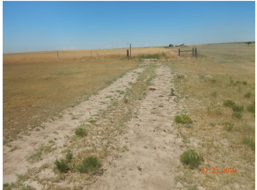
Photo 6: Photo taken from the access road, facing west. Photo shows access road has not been reclaimed.
