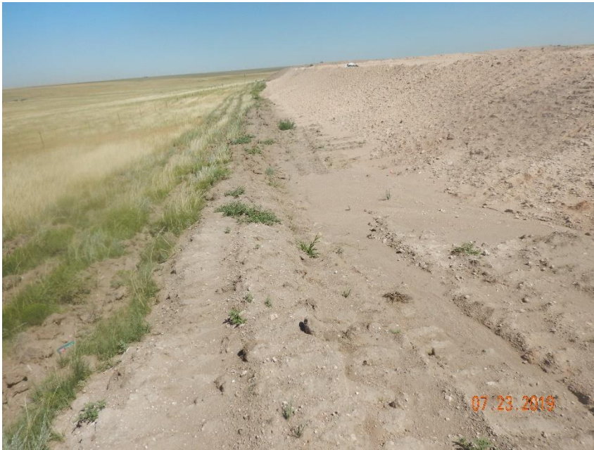
Photo 5: Photo taken from the west end of the location, facing north. Photo shows ditch/berm stormwater BMP, surface roughening (ripping) and tracking stormwater controls.
