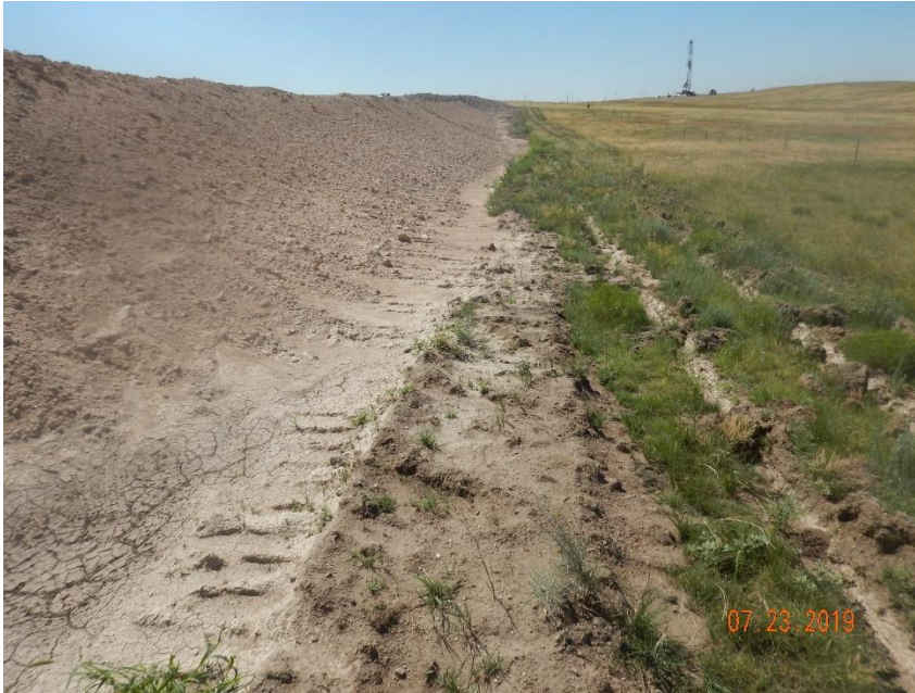
Photo 7: Photo taken from the northwest corner of the location, facing north. Photo shows stormwater erosion has filled the ditch with sediment. BMP requires maintenance.
