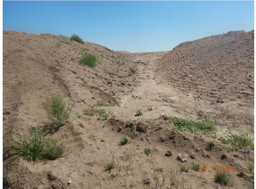
Photo 8: Photo taken from the northwest corner of the location, facing east. Photo shows erosion degradation evident between the pad and the topsoil stockpile on the northwest end of the location.
