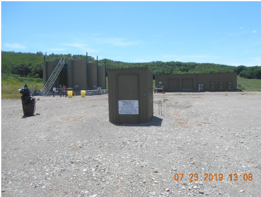
Injection wellhead inside housing.
