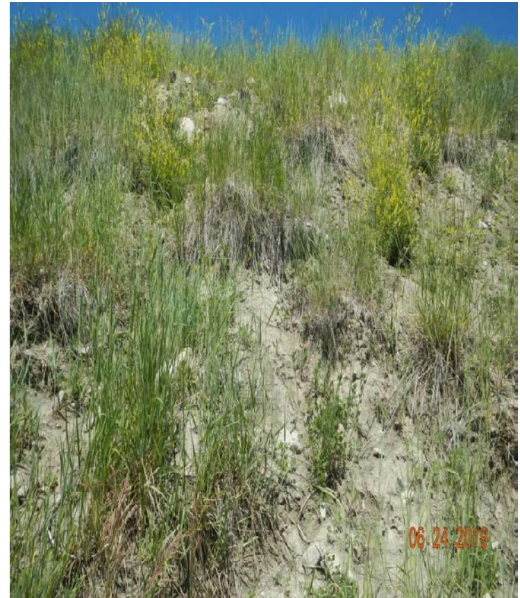
Photo#9: Fill slope has areas of spotty establishment of desirable vegetation.
