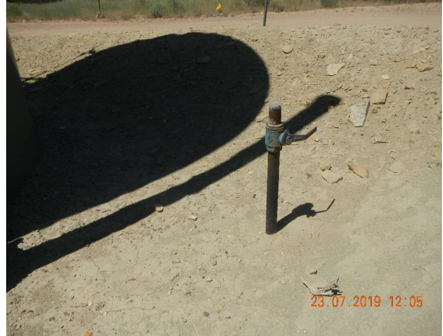
Photo #6 – View of the flowline located west of the tanks, within the secondary containment of the battery.
