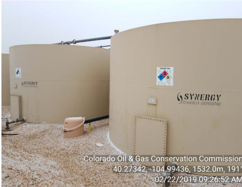
Crude oil tank placarding on 2/22/19
