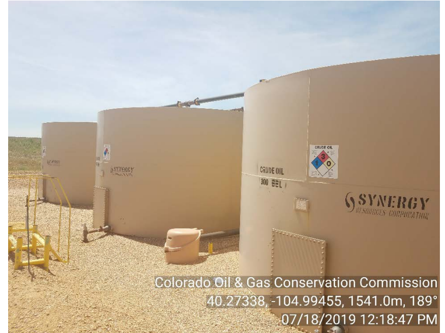
Crude oil tank placarding on 7/18/19
