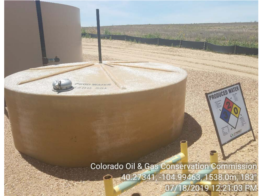
Produced water vault placarding on 7/18/19
