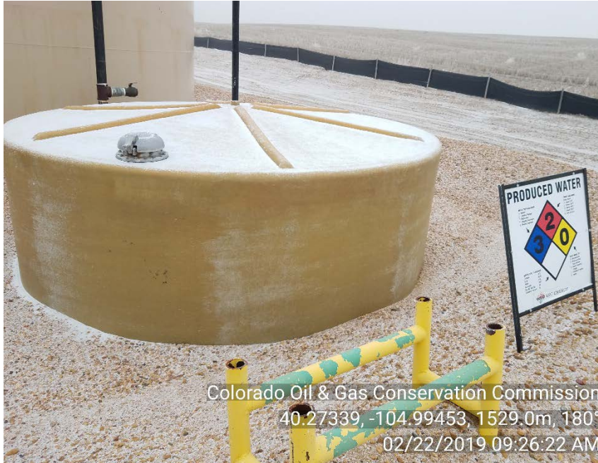
Produced water vault placarding on 2/22/19
