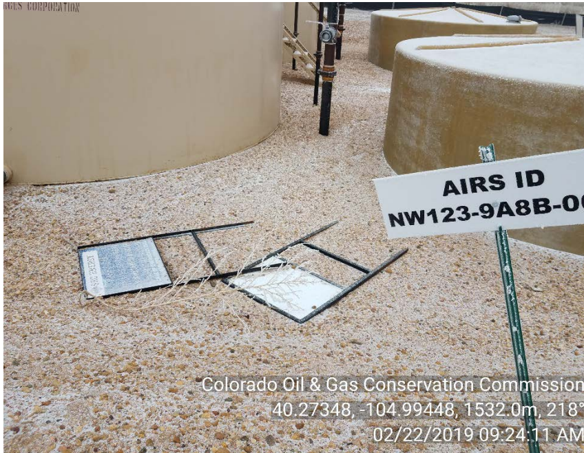
Unused equipment on 2/22/19
