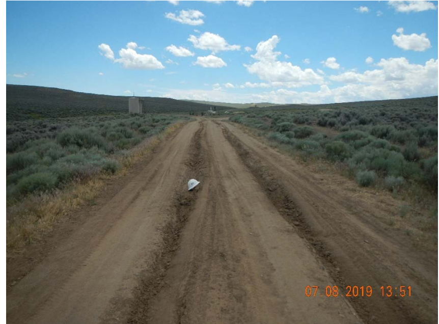
Photo 4. Rutting in access road. Hard hat for scale.
