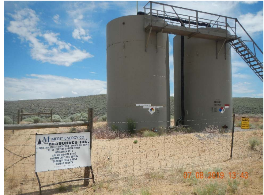
Photo 2. Merit Energy still listed as operator and with their emergency contact on battery sign. Weeds on/in tank battery.
