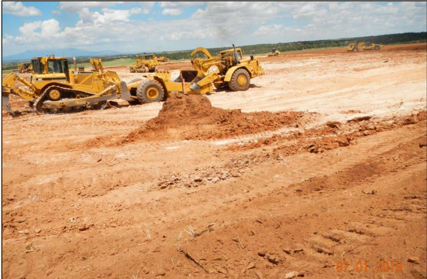
Photo 2. View of the well pad construction from the southeastern corner facing center. Well location staked.
