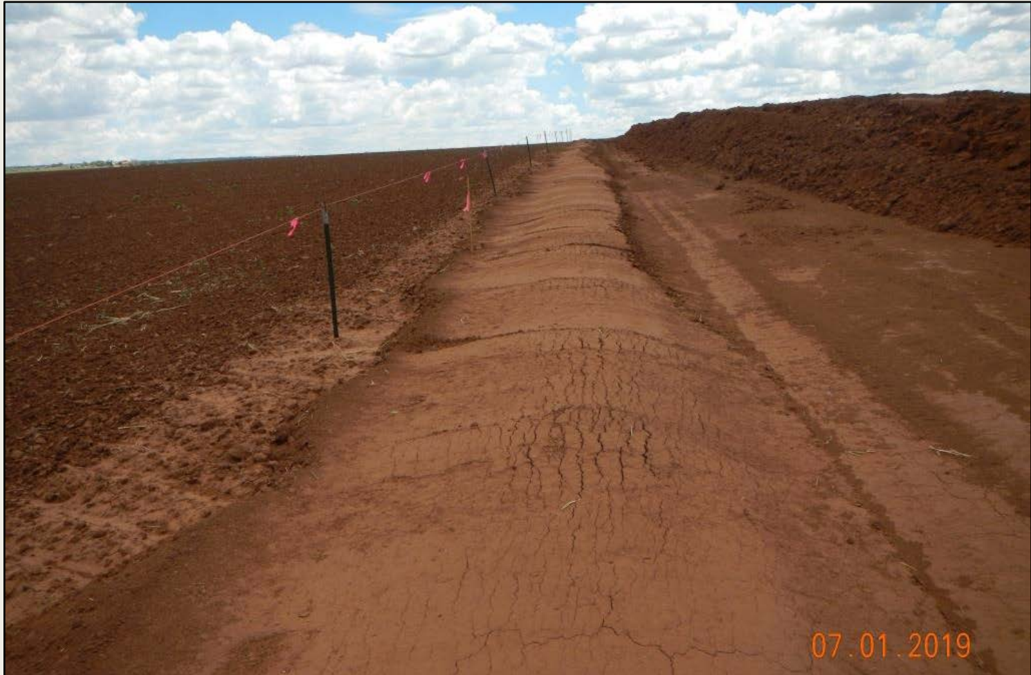
Photo 3. View of the northern edge of the project area. Compacted berm in place. Topsoil stored in northern project area.
