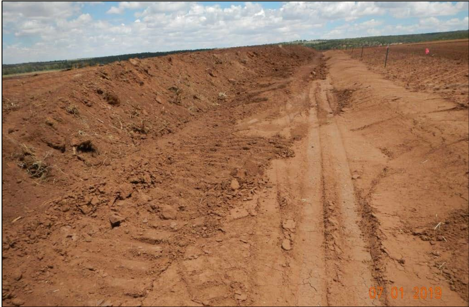
Photo 1. View of the eastern edge project area from the southwestern corner facing northward. Compacted berm in place around perimeter of disturbance areas. Topsoil stockpiled within.
