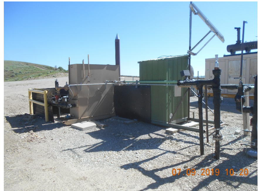
Separator and meter housing
