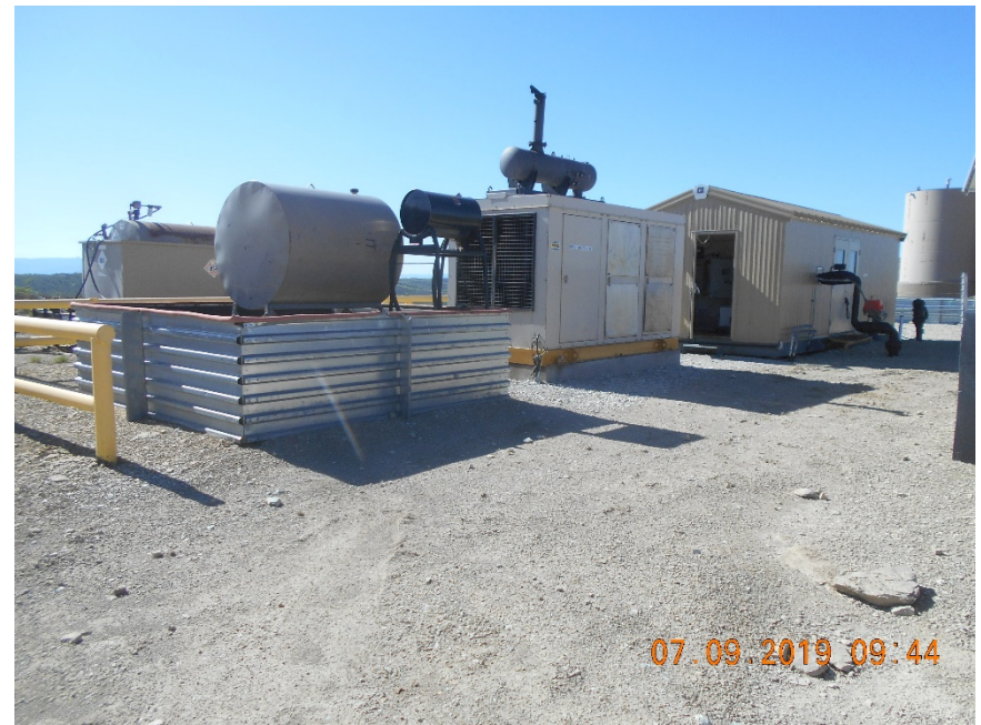
Pump Housing. Generator, fuel tank with secondary containment
