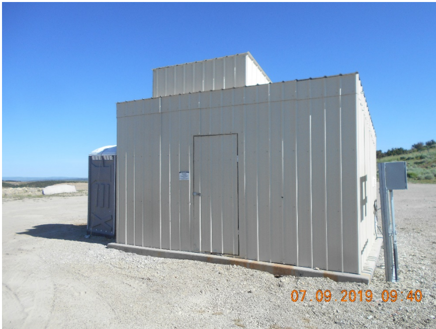
Injection wellhead inside housing.
