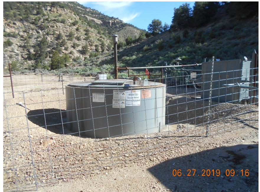
Blowdown tank with fencing and labels
