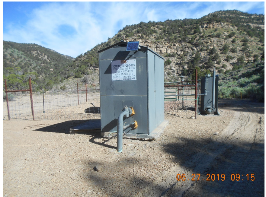
Meter housing with sign
