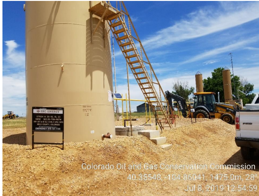
Photo 1: Centralized Tank Battery
