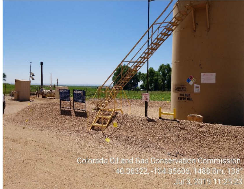
Photo 1: Centralized Tank Battery
