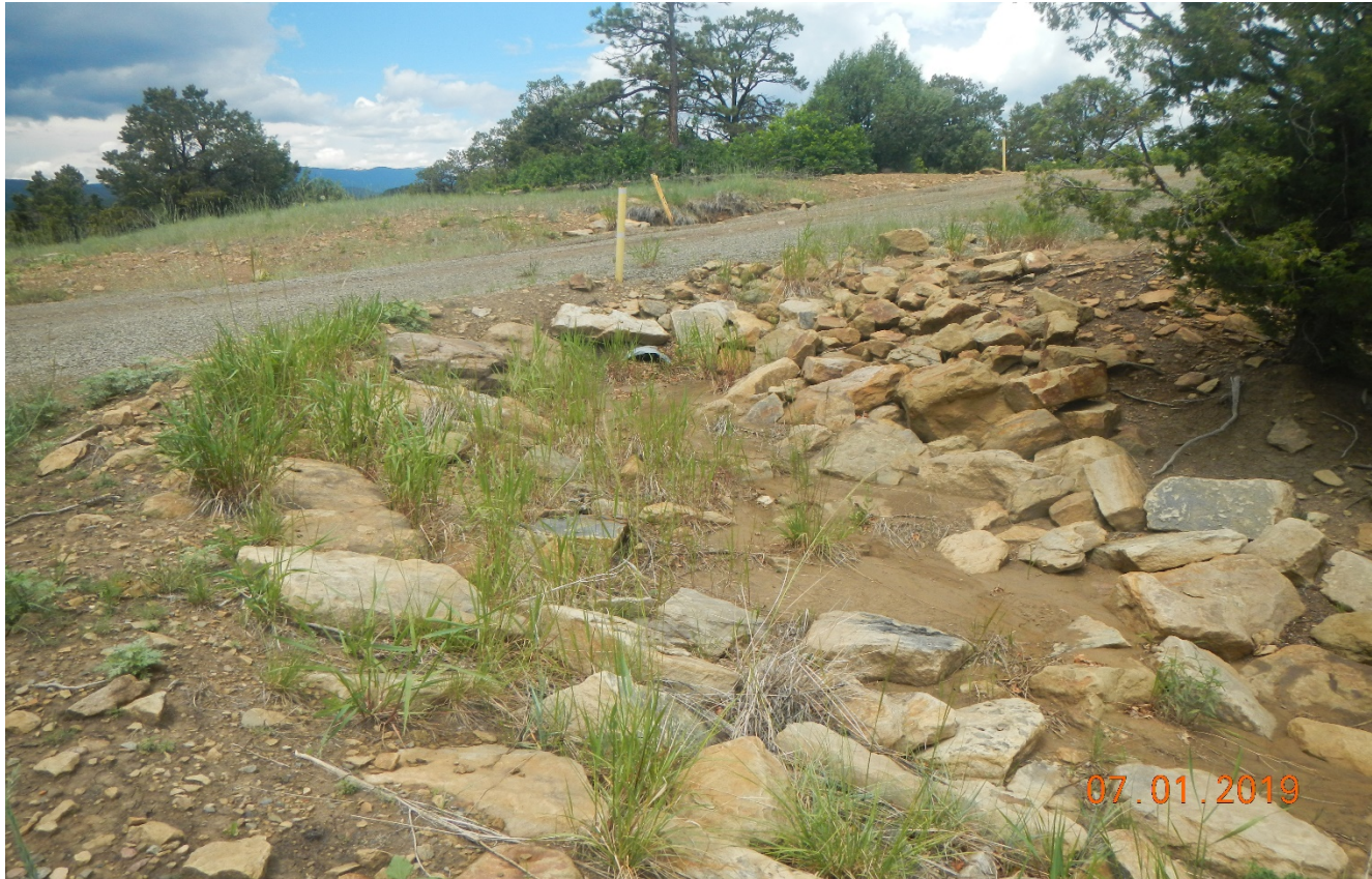
Photo 1. The culvert is full of sediment at outlet at the location. Did not check inlet.
