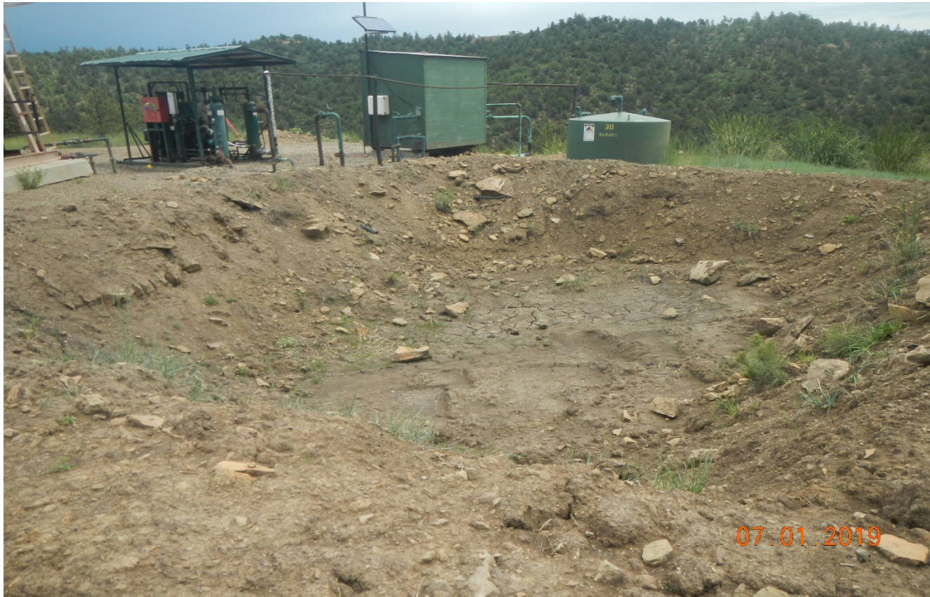
Photo 5. No freeboard marker was found in the pit.
