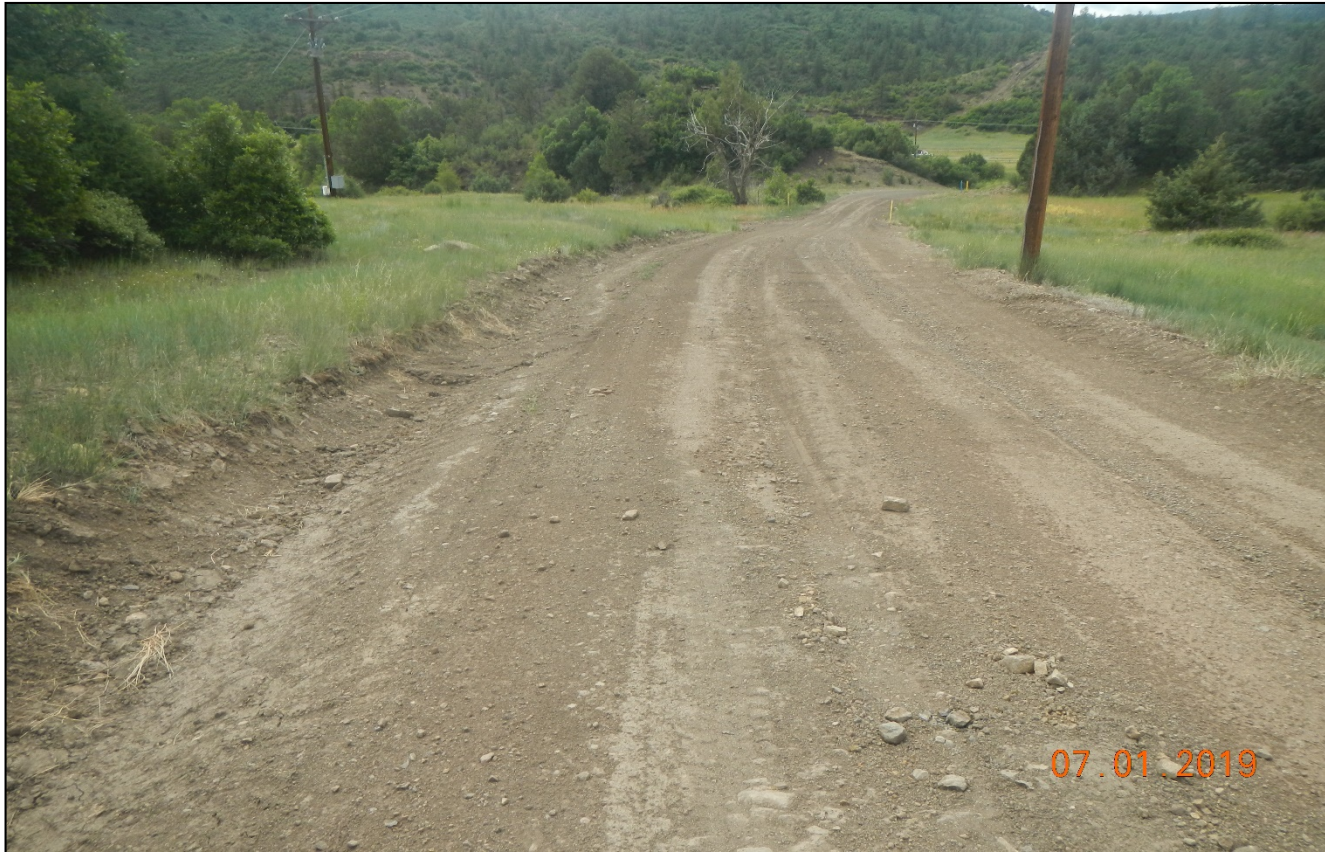
Photo 4. The side of the road has been regraded. The side may need erosion controls to prevent erosion. (e.g. check dams)
