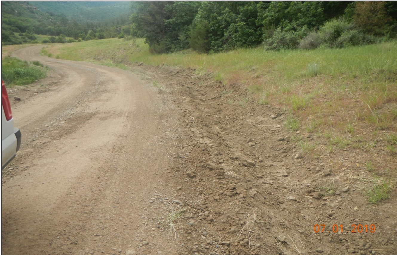
Photo 5. The erosion channel at the southeast side of the location has been repaired. The area may need erosion controls to prevent erosion. (e.g. check dams)
